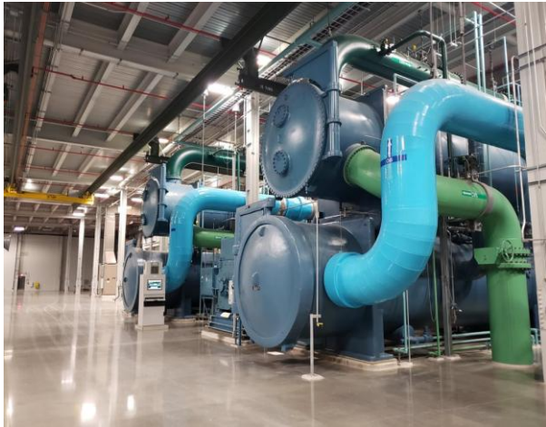
Figure 5: Water chiller connection
